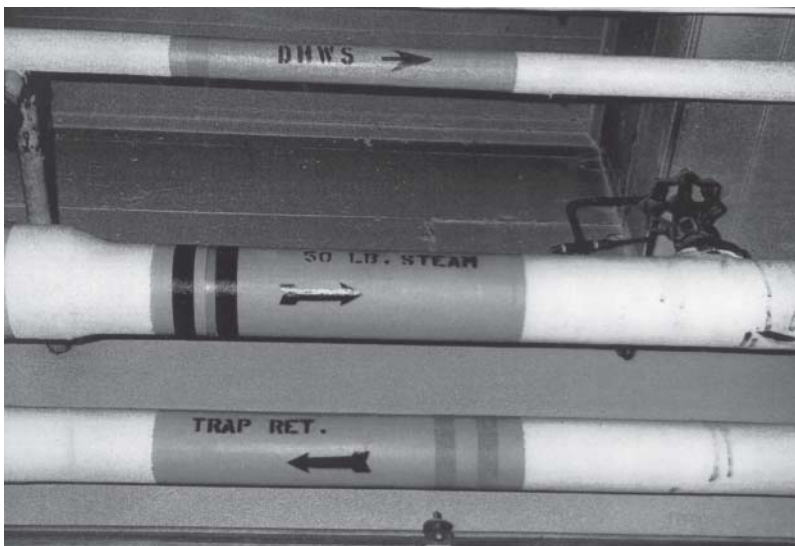
Controlled products in pipes identified by colour and letters.
